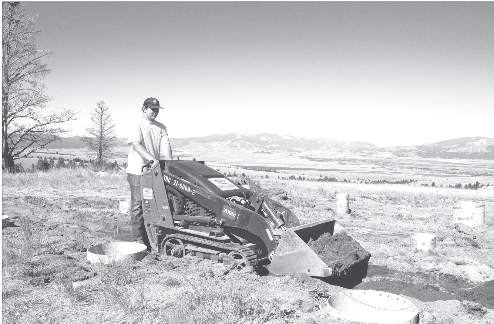
Bridger Johnston of Anaconda is pictured working for Crummer Construction LLC under the American Jobs for America's Youth Summer Jobs Program in 2022. Courtesy photo.
